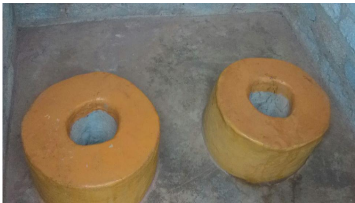
Picture: Toilet in an unregistered ECD in the North Region
